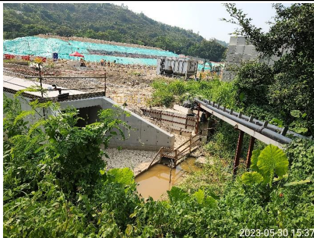
(P1) Water (upstream river water and site runoff) detained near the box culvert.
