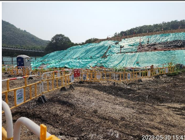
(P3) Slope was covered by tarpaulin sheets to minimize muddy runoff under rainfall.
