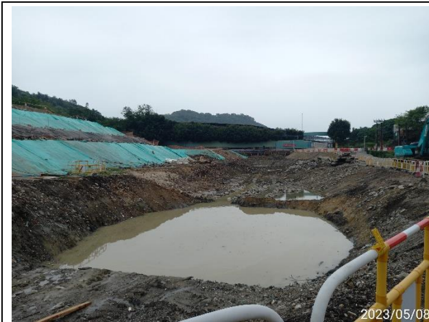
Temporary detention pond at the works area near the access road (R1)
