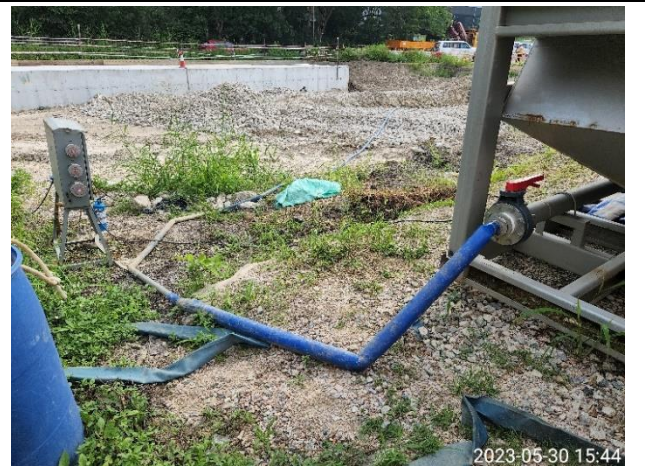
(P2) Water detained within the sump was directed to the WetSep by a drainage pipe.
