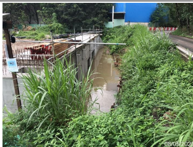
Water (mixed upstream river water and site runoff) detained temporarily behind the box culvert prior to treatment (R3)
