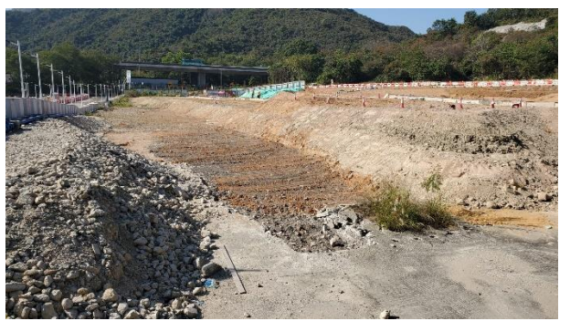
No muddy surface runoff and direct effluent discharge was observed during site inspection.
